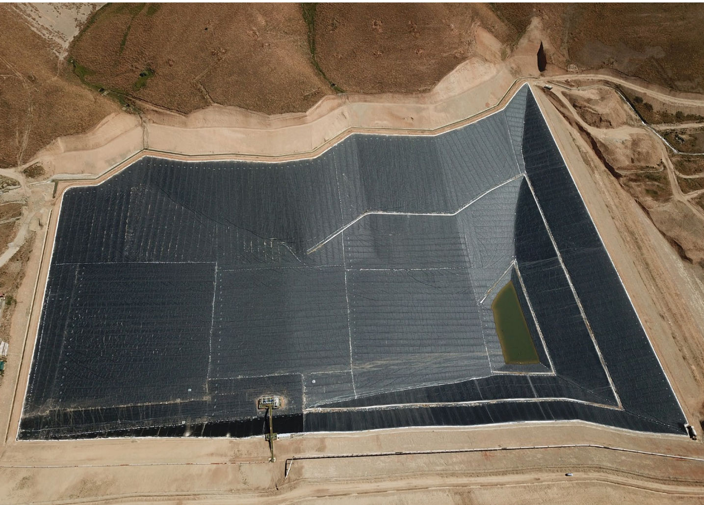
FIGURE 8 A tailings dam project at Chaarat Mine, Kyrgyzstan. Photo courtesy of ATARFIL.
