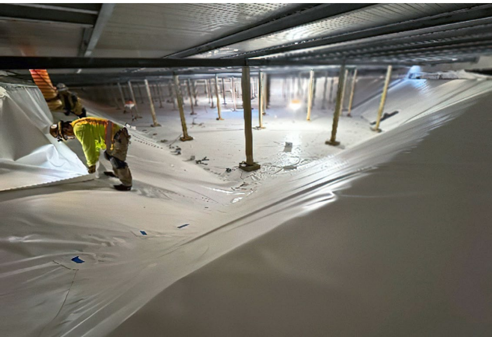
FIGURE 7 Seaman Corporation's 9146 XR-PW geomembrane potable water storage renovation at Thunderbird Reservoir in Phoenix, Ariz. Photo courtesy of Field Lining Systems Inc.
