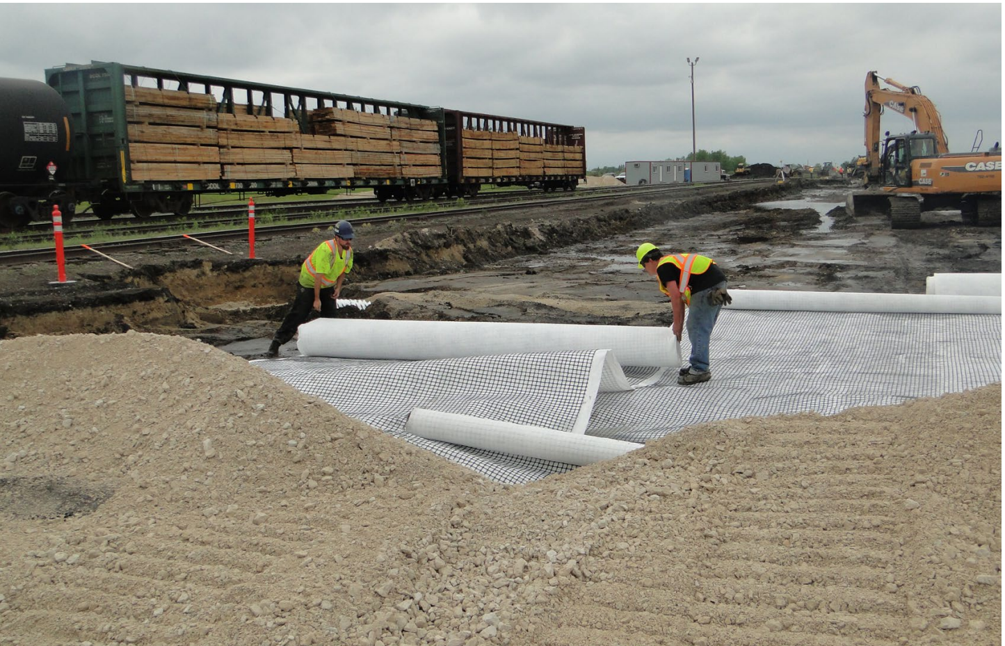
FIGURE 6 Here, the Swamp Grid™ from Titan is being deployed at the Transcona railyard in Winnipeg, Man., Canada. The Canadian National Railway wanted an additional six-track extension at the yard; a challenge since the site was swampy, with wet and soft clay soils. The biaxial Swamp Grid, consisting of Pyramid Grid™ bonded to a six-ounce continuous filament, needle-punched nonwoven geotextile provided the solution. Photo courtesy of Titan Environmental Containment Ltd.
