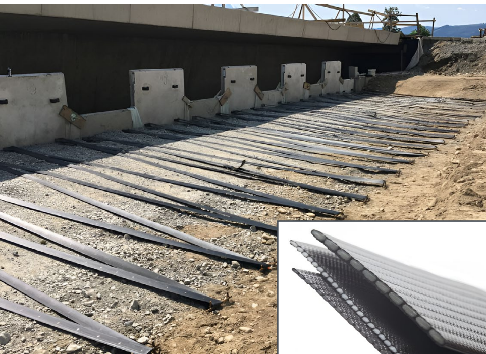
FIGURE 4 Designed for reinforcement applications in combination with concrete wall facing panels, the ParaWeb geogrid from Maccaferri is being used here as a geogrid reinforcement layer for a concrete panel facing a MSE (Mechanically Stabilized Earth) wall.
