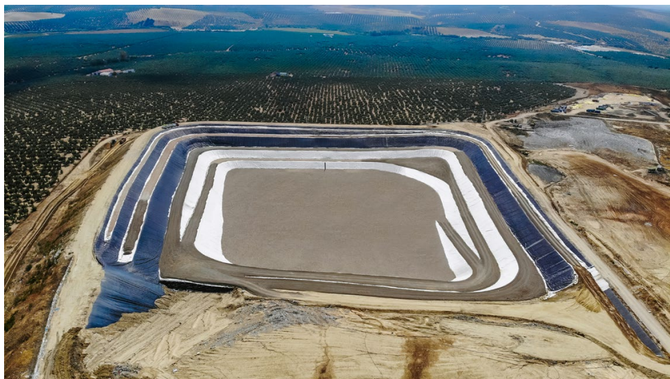
FIGURE 9 A municipal solid waste landfill cell extension project in Cordoba, Spain. Photo courtesy of ATARFIL.
