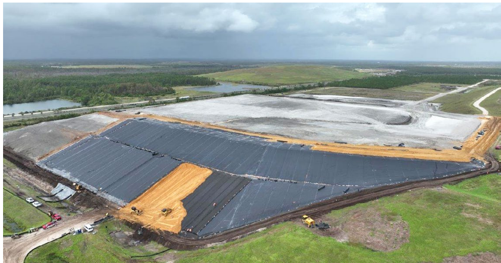
FIGURE 10 Phase 1 of the Orlando Utilities Commission's coal ash landfill closure as part of a project to create a renewable energy facility in Orlando, Fla. Photo courtesy of ATARFIL.
