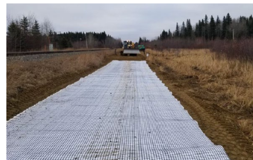
FIGURE 8 Railway track beds running from Edmonton to Edson, Alta., Canada, needed to be twinned, a project taking place during the winter and over poor soil conditions. Titan deployed its Swamp Grid 30 geogrid as a means to stabilize the railway track bed, utilizing a three-lift design, with each lift including one layer of the geogrid along with gravel. Photo courtesy of Titan Environmental Containment Ltd.
