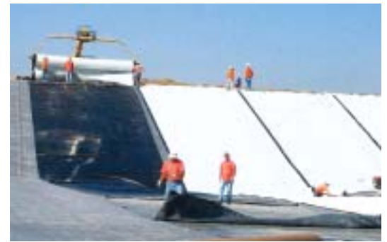
Photo 4. Thorough testing by manufacturers during product development and CQA personnel in the project design phase helped make the Visalia Landfill project, with its geosynthetic mix, a success.
