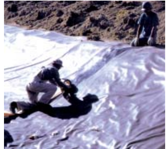
Photo 3. With water loss exceeding replenishment, irrigation districts are turning to canal liners. Geomembranes, either on their own or combined with concrete linings, perform extremely well.
