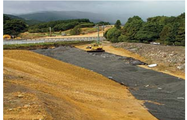
Photo 2. A combination of geogrids and wick drains improved the stability of site soils, creating a safer stretch of road.
