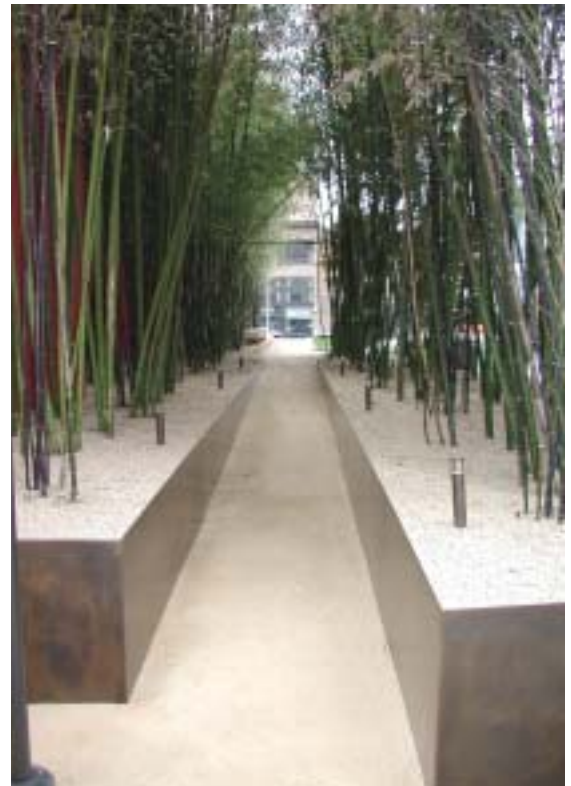
Photo 1. Specifications called for a root barrier sheet, a prefabricated drainage course, and filter fabric to ensure proper conditions for the bamboo grove.
