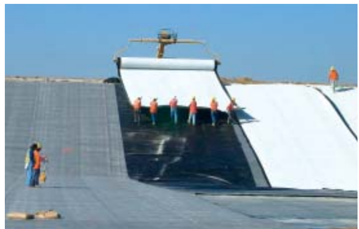
Photo 2. Textured HDPE being installed over GCL with the use of a slip sheet.
