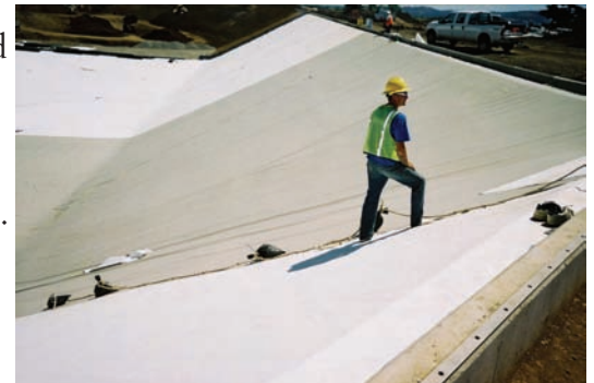
Photo 3. The 100-million gallon facility provides Salem with two-thirds of its drinking water. Following liner installation, a polypropylene floating cover was added to insure against contamination.
