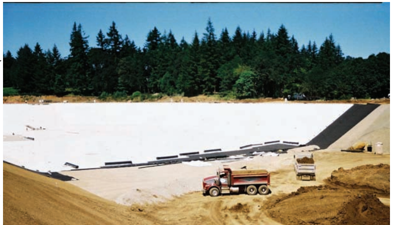
Photo 2. Earthwork operations can greatly affect the success of a liner installation. At the Franzen Reservoir site, the grading and ground preparation were exceptional.
