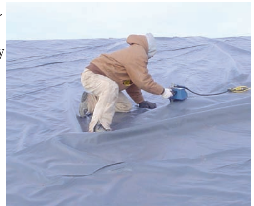
Photo 2. Cold-weather seaming is difficult because the material is at risk for stiffening, wrinkling or folding. Geomembrane rolls were stored in a heated trailer on site until it was ready for deployment.
