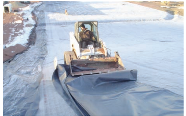
Photo 3. Large panels of PVC were fabricated in the factory to reduce the field work. This was especially important given the weather conditions. The prefabricated panels were larger than normal.
