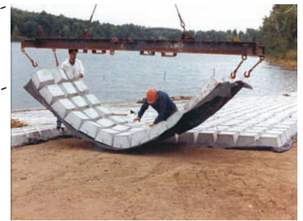
Photo 2. Flexible "cable concrete" being installed. A geotextile sheet is fused to the underside. Its separation characteristics provide drainage and stability to subsoils.
