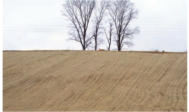
Photo 1. Here today, gone tomorrow: Totally degradable erosion control blankets are being specified on a wide-scale. Project managers like the quick establishment of vegetation, and clients are drawn to the “green design.”
