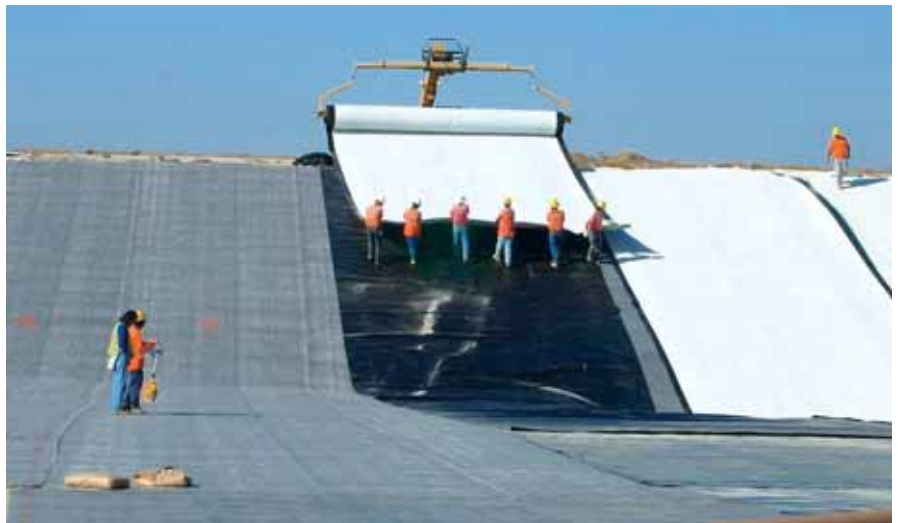
Photo 1. Textured high-density polyethylene (HDPE) geomembrane being installed over a geosynthetic clay liner (GCL) with the use of a slip sheet. Landfill projects like this, if left to inexperienced teams for the sake of a lowest overall bid, present serious safety and financial risks.
