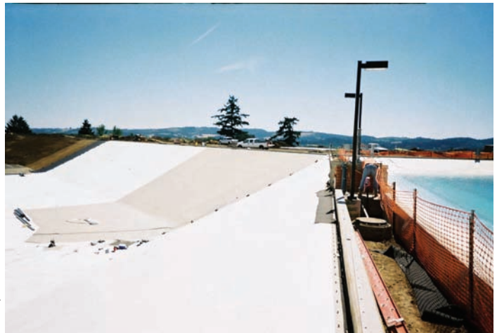
Photo 1. Dividing the reservoir in two allows partial draining of the reservoir, if needed, without interrupting overall service.
