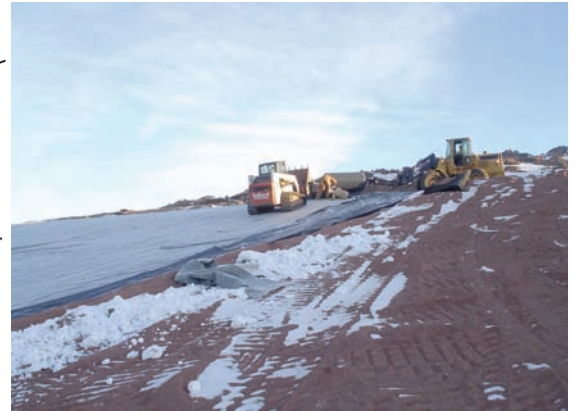
Photo 1. Winter installations are rarely welcomed, but the county had no choice. The county's landfill had reached capacity.
