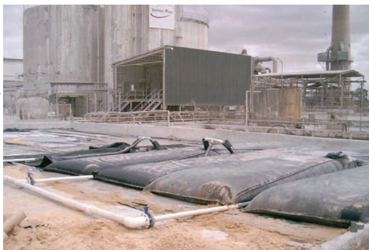
Photo 1. The switch to woven geotextile bags for sludge solids removal enabled secondary conditioning to begin after two weeks when previously the facility operators had to wait up to six months.
